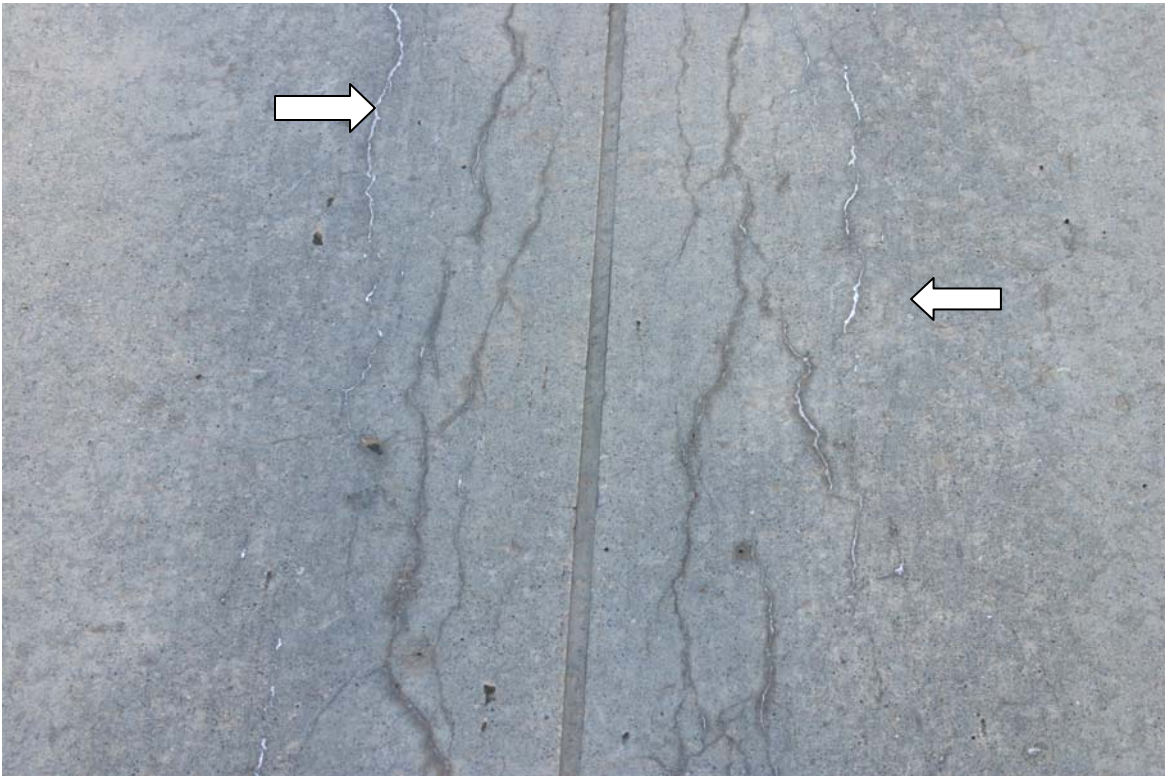
Figure 3. Cracking with white ASR exudate (arrows) in cracks.
