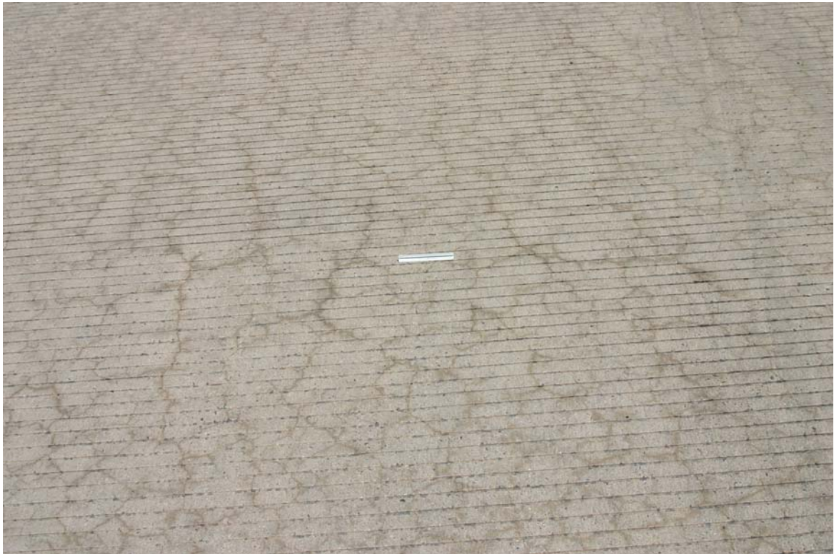
Figure 1: Pattern cracking observed in a concrete pavement due to ASR.
