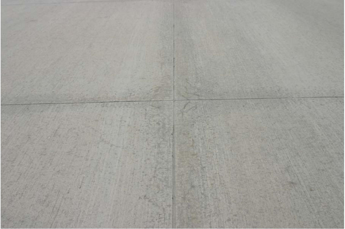
Figure 2: Cracking concentrated at joints in a concrete pavement due to ASR.
